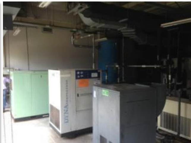
Air compressor plants (3units)
