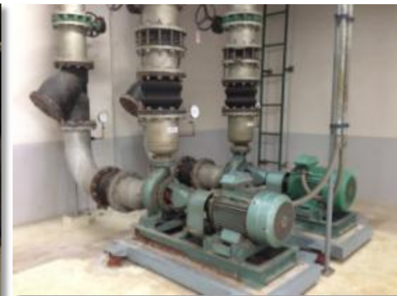
Condenser Water Pumps (22kW x 2 units)
