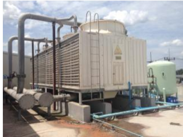
Cooling tower (450 tons x 3 units)
