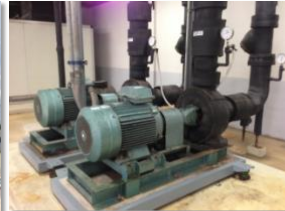
Chilled Water Pumps (45kW x 2 units)
