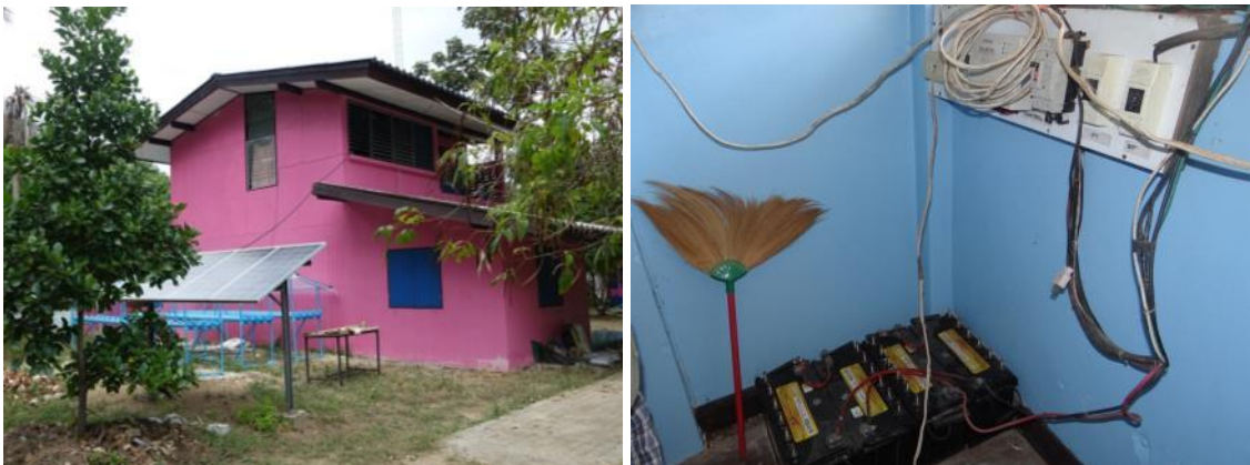
Figure 18: PV-battery system supplying the building for teacher resting
