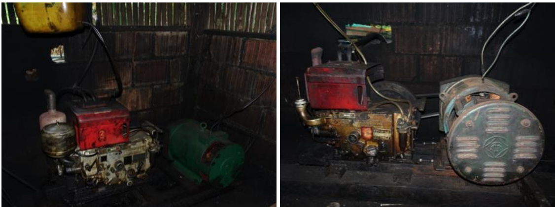
Figure 9: Generator #18a and #18b owned by Chaolae Homestay
