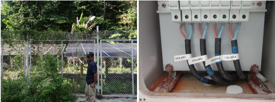
Figure 21: PV system supplying the electricity for the BTS1 (PV1) and rusty components
