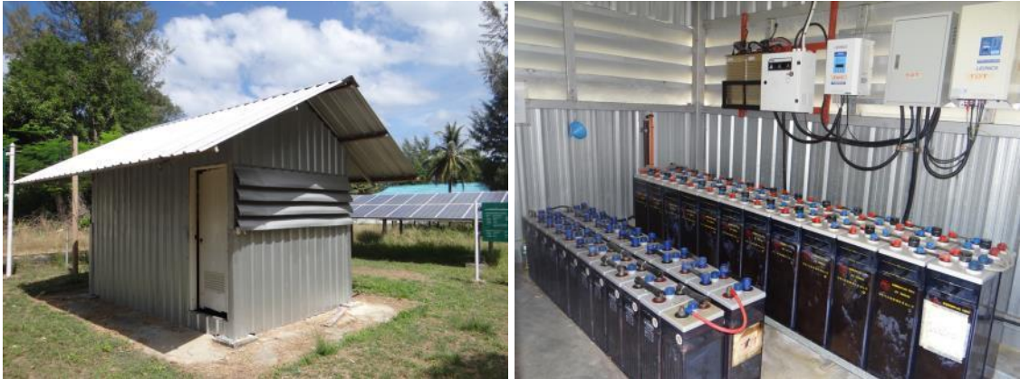
Figure 14: Power house including charge controller, inverter and batteries
