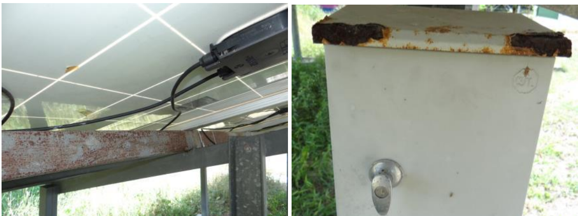
Figure 16: Rusty mounting structure [left] and combiner box [right]
