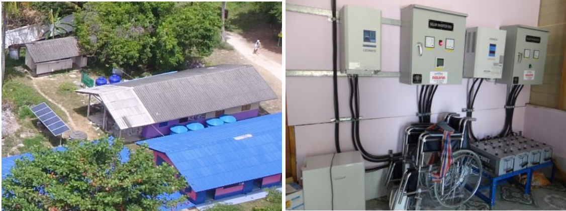
Figure 17: PV-battery system supplying public health centre
