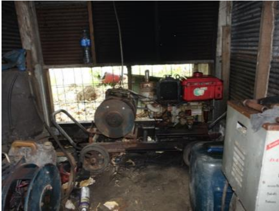
Figure 8: Generator #12 owned by Mr.Sompong
