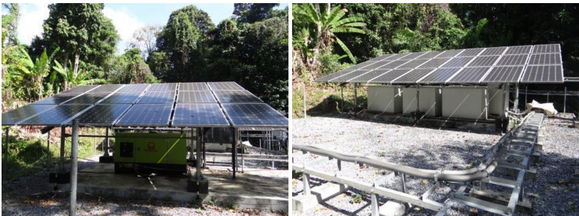
Figure 22: PV system supplying the electricity for the BTS1 (PV2)
