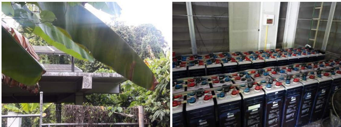
Figure 25: PV rooftop and batteries supplying BTS2
