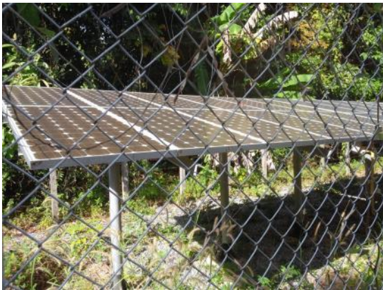
Figure 42: Twelve broken SHARP modules at BTS1
