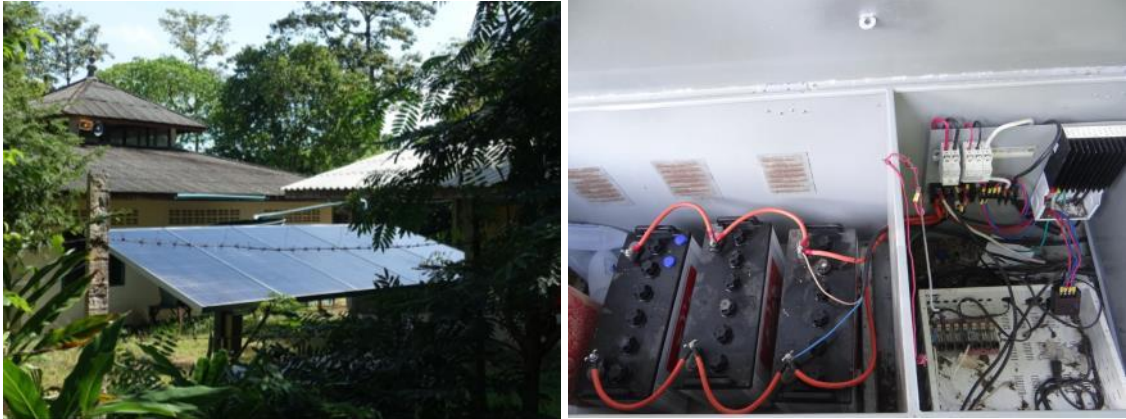
Figure 26: PV system located at mosque
