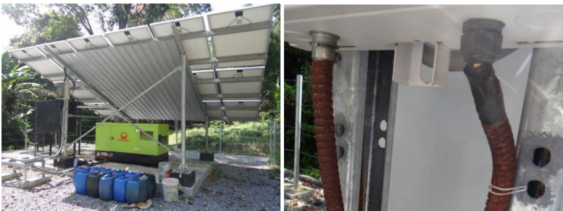
Figure 23: Poor ventilation for PV modules [left] and rusty flexible conduit [right]
