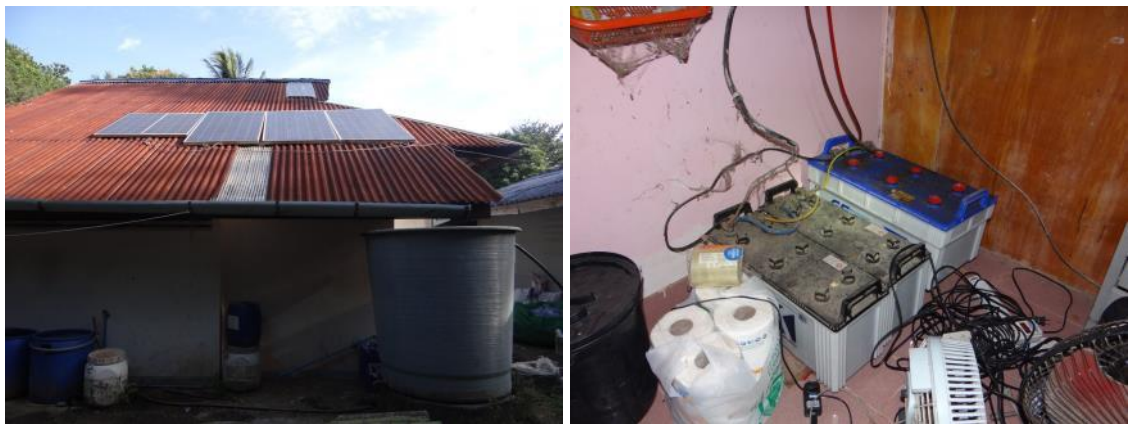
Figure 12: Solar Home System with batteries
