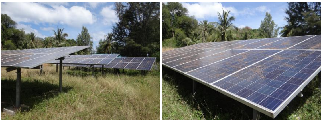
Figure 15: Dirty PV modules observed
