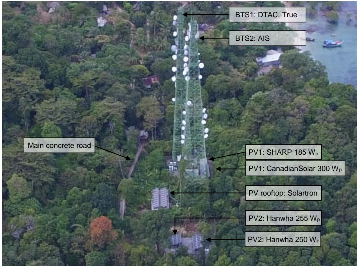
Figure 19: Overview of BTS1 (True,DTAC), BTS2 (AIS) and PV systems
