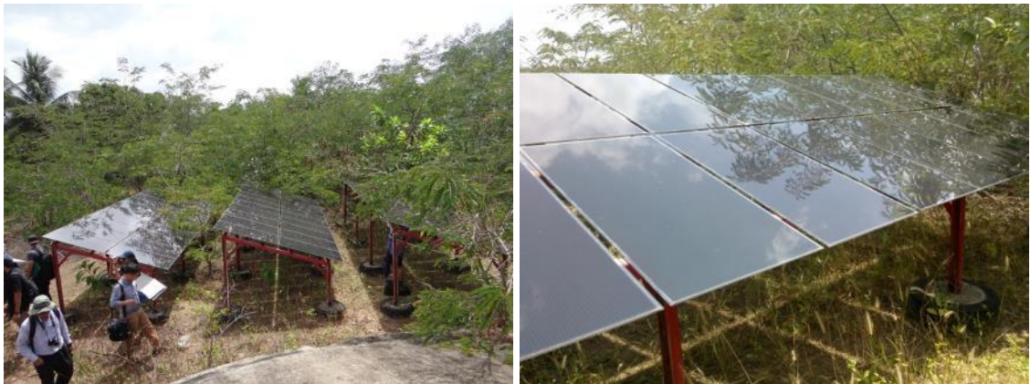
Figure 14: 3 kW p PV system located next to water storage
