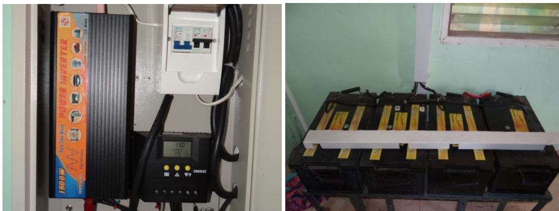
Figure 22: Inverter and charge controller [left], four Globatt batteries [right]
