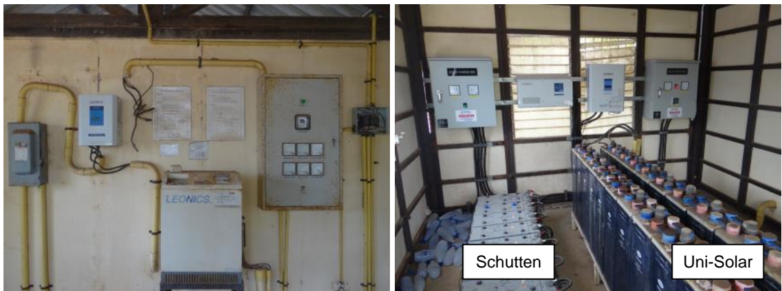
Figure 18: Inverter and batteries system inside powerhouse
