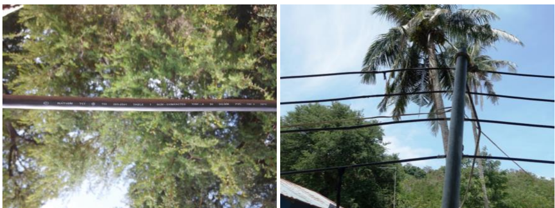
Figure 28: THW 50 mm 2 cable (Existing central grid transmission line)
