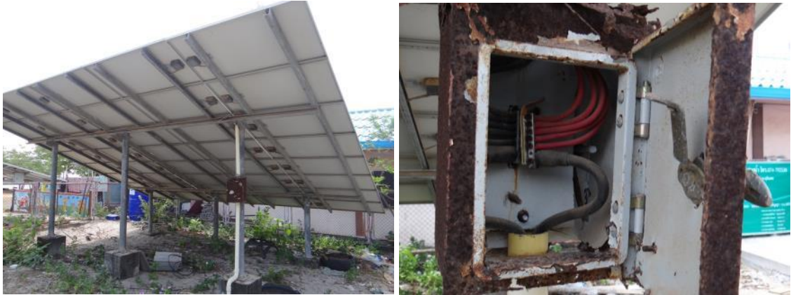
Figure 19: Rusty combiner box
