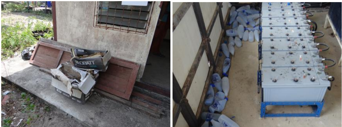
Figure 20: Unorganized garbage in the powerhouse
