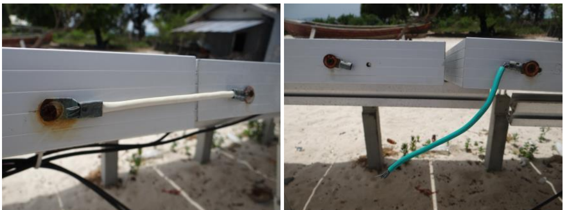
Figure 25: Rusty screws [left], disconnected grounding cable [right]
