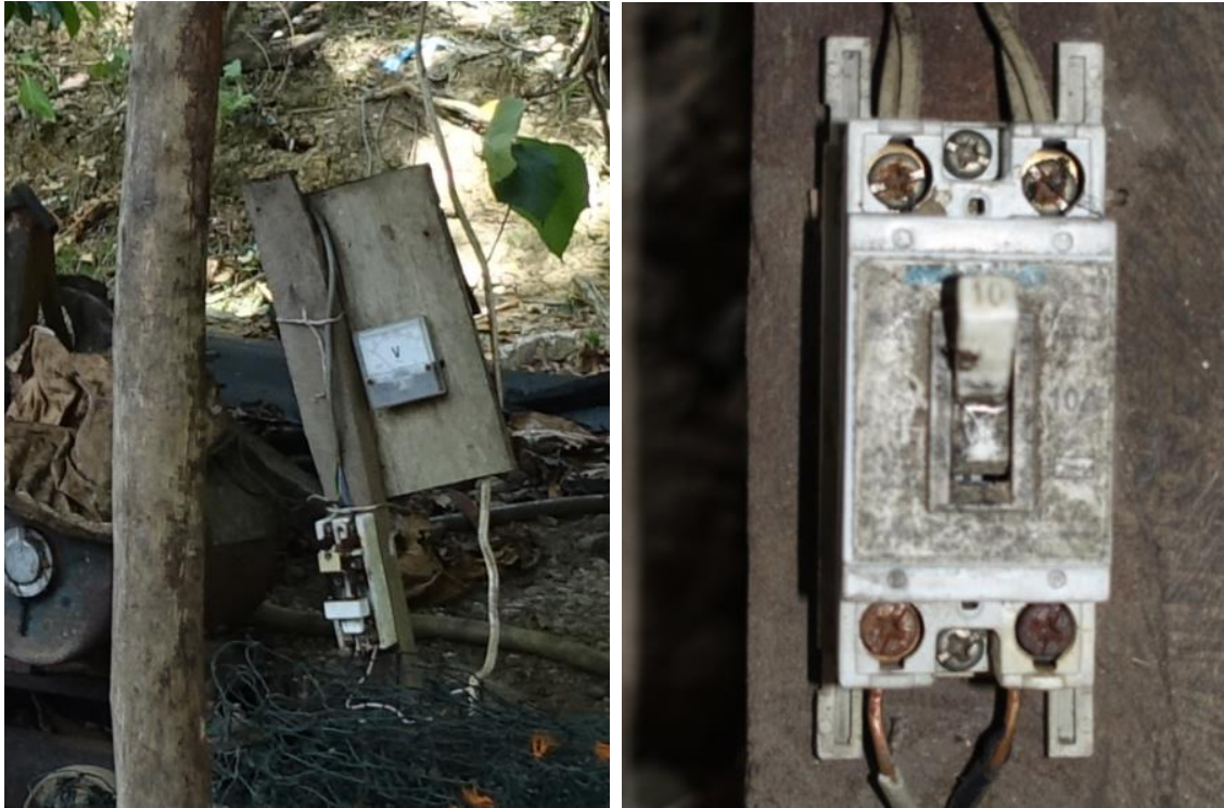
Figure 35: Disconnect Switch and Circuit Breaker for Generators
