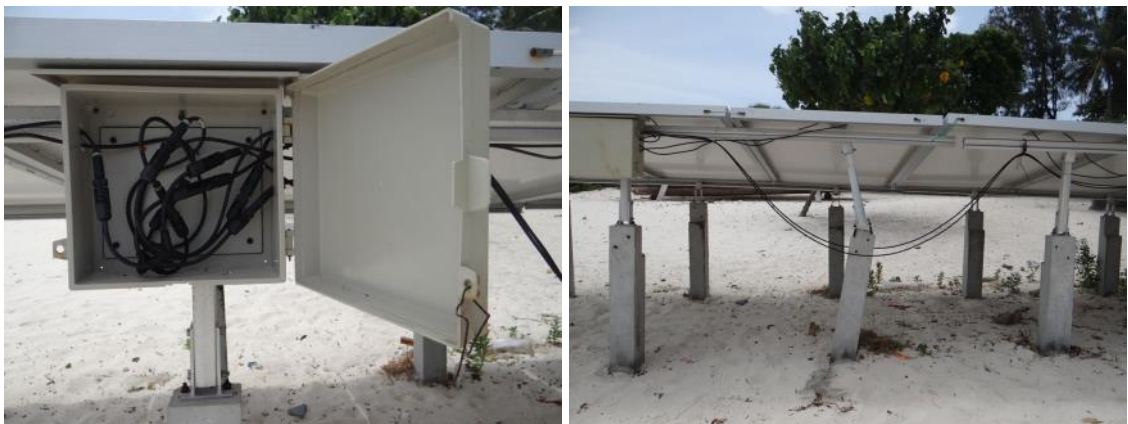
Figure 24: Untidy combiner box [left], damaged mounting structure [right]
