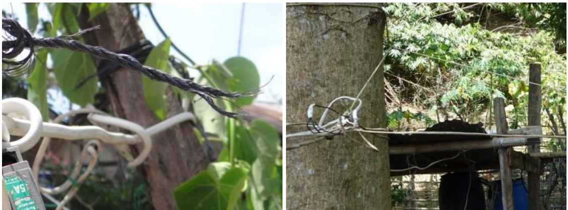
Figure 34: Wooden pole and tree connection of private connections
