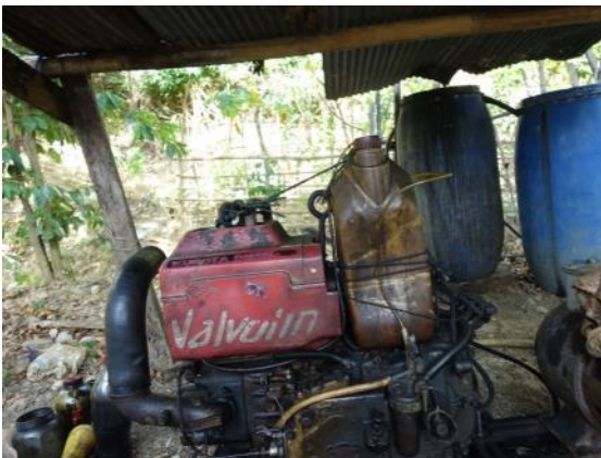
Figure 8: Generator #33 under a small roof of welded brass
