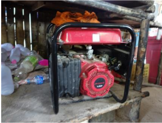
Figure 11: Generator #40 in a small shop/restaurant under metal sheet roofs
