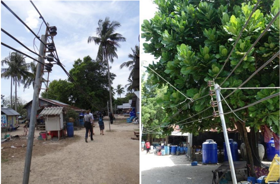
Figure 33: Steel pole of main grid
