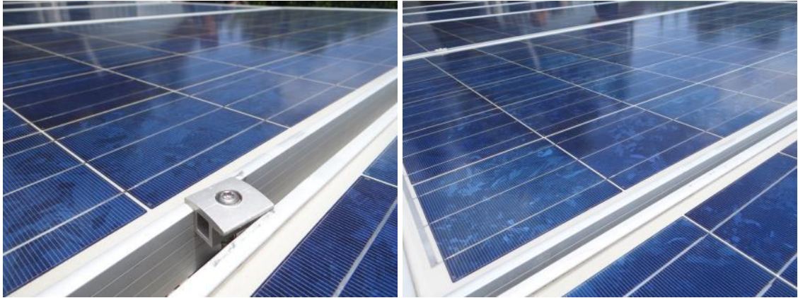
Figure 23: loose clamp [left], missing clamp of PV module [right]
