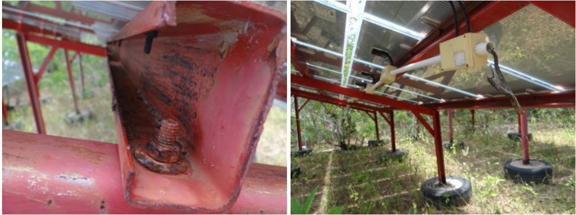
Figure 16: Rusty metal [left] and disconnected cable [right]
