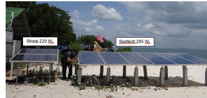
PV system @ public health centre 220 Wp ( not working ) + 1.71 kWp (working)
