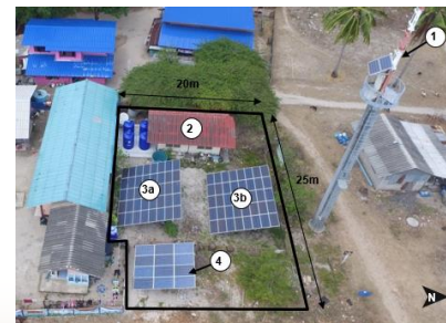
PV system @ School 5.12 kWp ( not working ) + 3.0 kWp (working)
