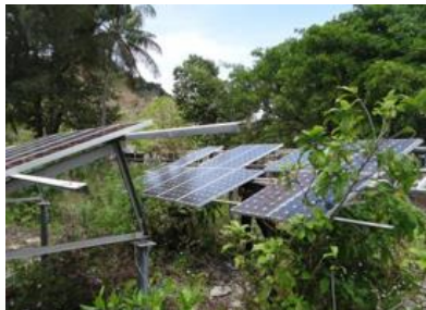
Abandoned PV system @ beachfront
