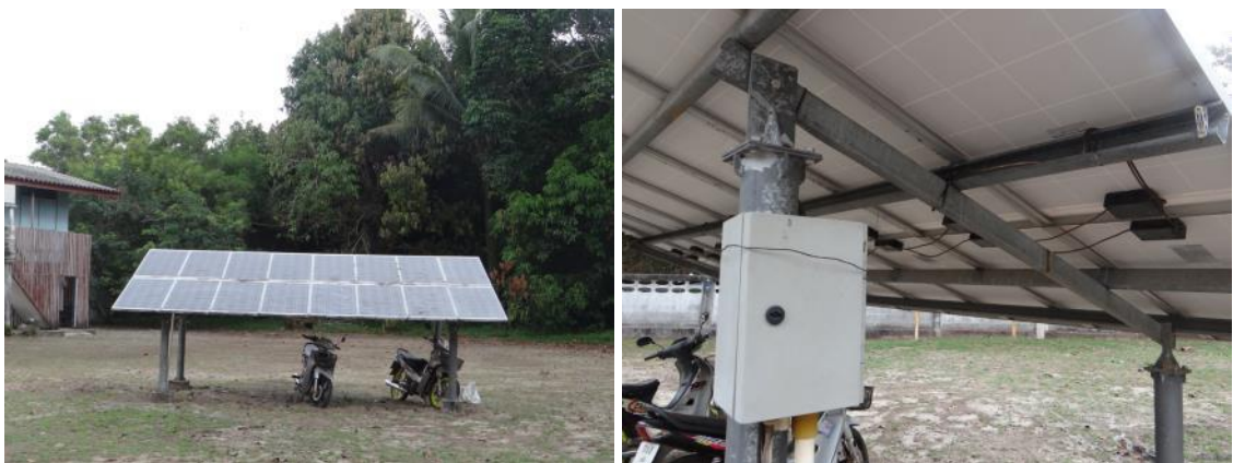
Figure 15: 2 kW p PV system powering the public health centre
