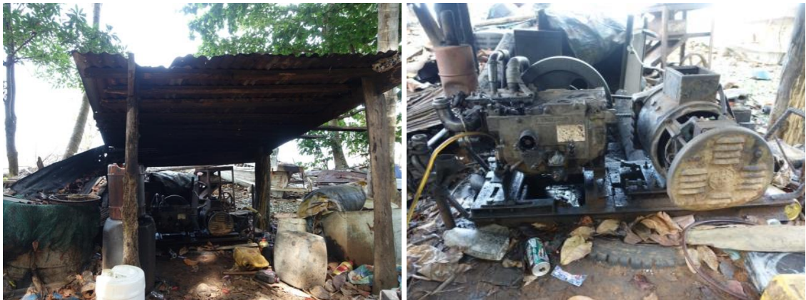
Figure 6: Generator #62 under the corrugated sheet roof
