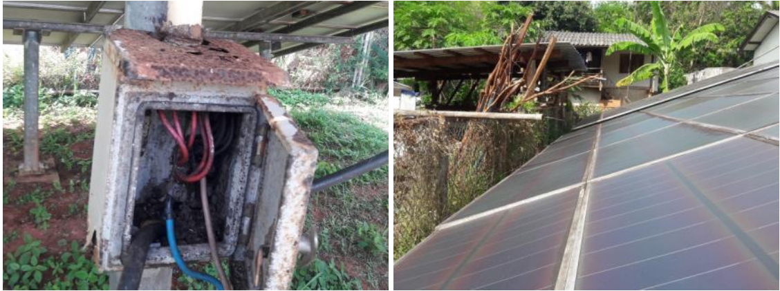
Figure 14: Rusty combiner box and thin film modules
