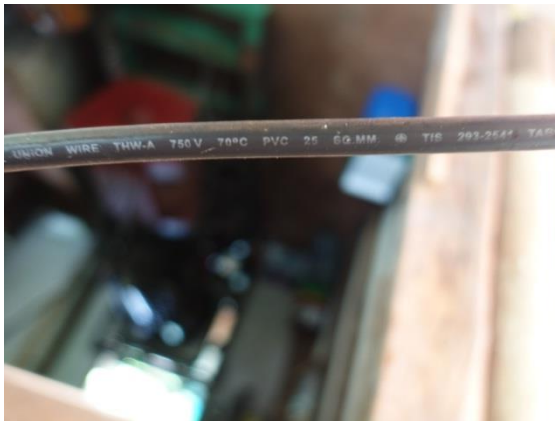
Figure 21: 25 sq.mm THW–A cable in Grids of Generator #40 and Generator #41
