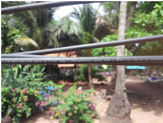
Figure 23: Cables in Grid of Generator #68
