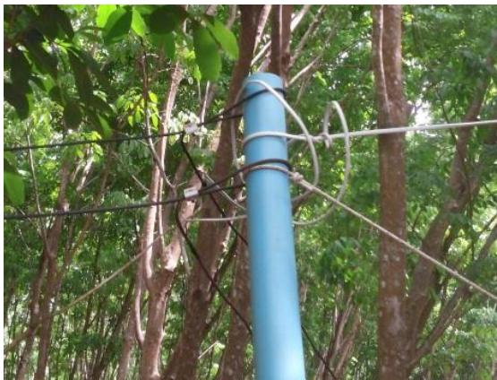
Figure 20: VAF cable (white cable) connected with THW-A cable (black cable)
