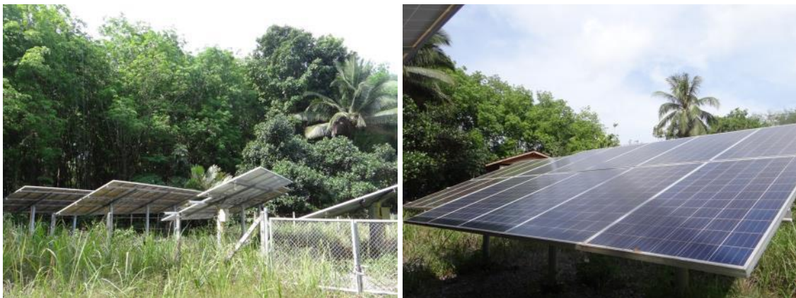
Figure 11: PV system at BTS
