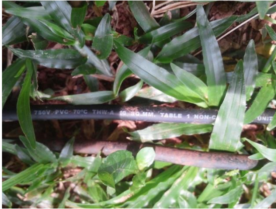
Figure 24: Cables in Grid of Generator #66
