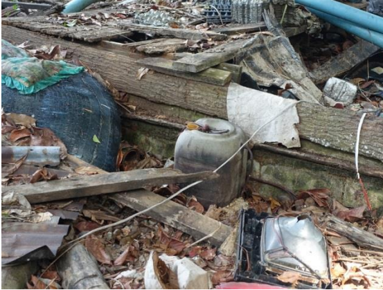
Figure 27: Ground lying cable transmission connected to Generator #62 (white cable)
