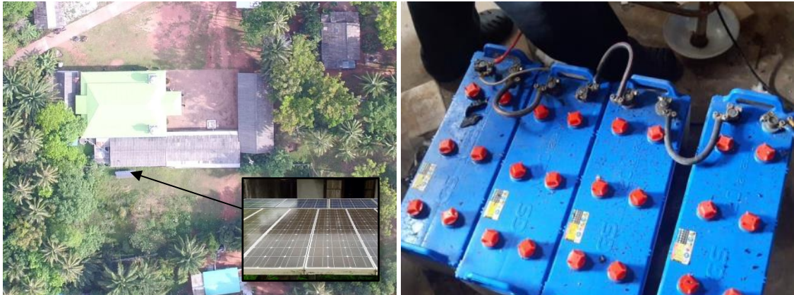
Figure 10: PV-Battery system supplying the electricity for the mosque
